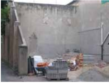
The derelict site at the rear of the College is to be transformed into a Meditation Garden.
